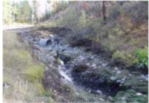
Above: storm flows overwhelmed stream channels and culverts
