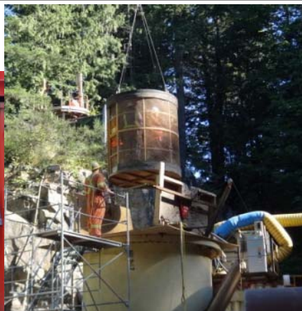
Vancouver Coastal's intrepid explorers being lowered into the shaft that leads to the water tunnel
