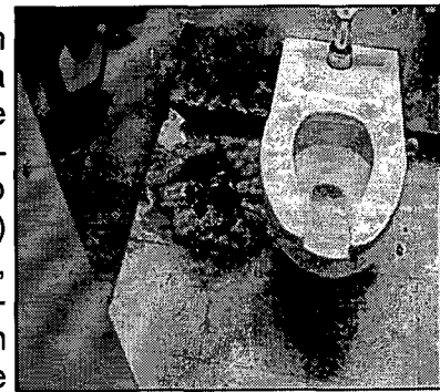
Sewage backed up from drain
