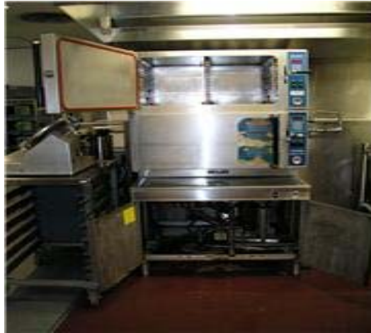
An acceptable modified non direct steam box . Note the heat exchanger underneath.
