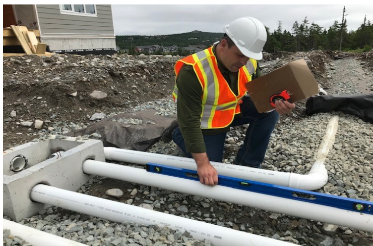
Photo Credit Tammy McDonald. Chris Hart, EHO, actively inspecting a sewage disposal system
