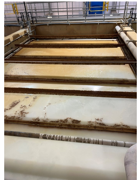
Combined DAF and filtration basin at Powers Creek.
