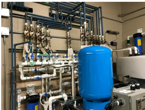
Figure 2 - Potable water treatment system within a building (Passed inspection)
