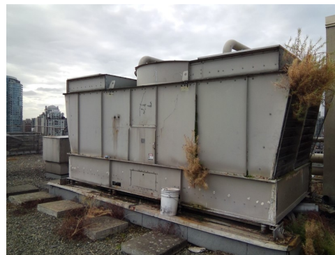
Figure 4—Cooling Tower (Did not pass inspection)
